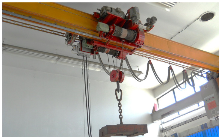
Figure 1: Single girder bridge crane
